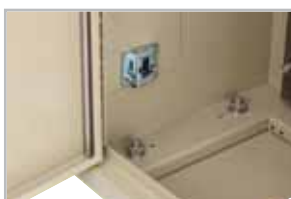
cable entry door (inside)
